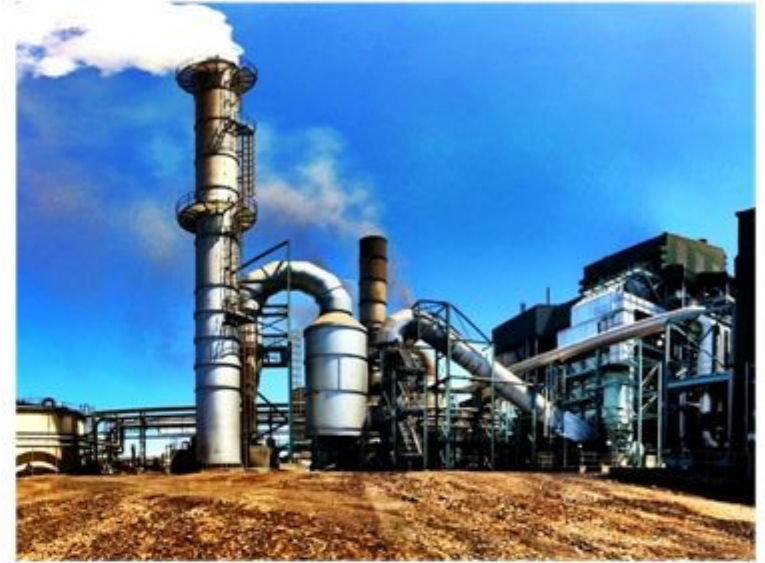
Ubombo Sugar Mill – Boiler No. 8
